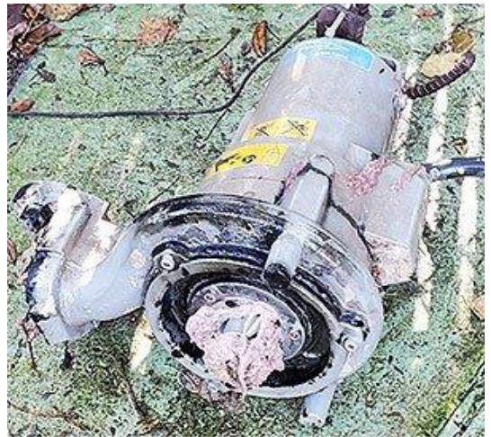
Lift Station Clogged With "flushable" Wipes
